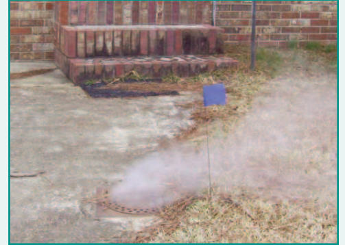
Smoke testing is a critical step during the Sanitary Sewer Evaluation Study (SSES) to identify possible incidents of Inflow and Infiltration within the MWA system.
