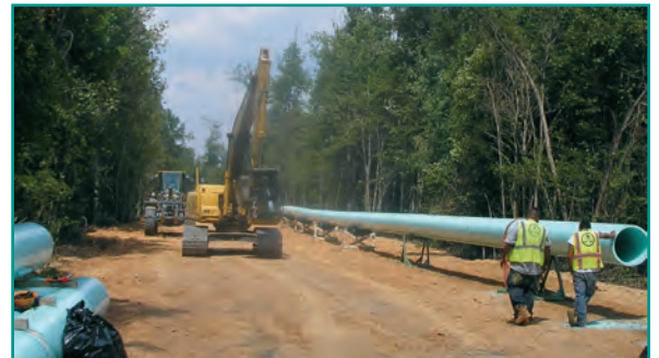
The MWA “Allen Road II Lift Station and Force Main” project involves the installation of a 24-inch force main underneath a wetland that is nearly a mile wide, without disturbing that natural resource during construction.
