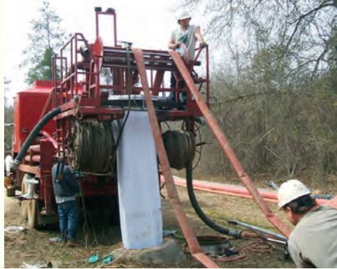
Among four current capital improvements to the MWA sewer system is a major project investing more than $3 million in pipe lining (shown here) and rehabilitation of sewer lines and manholes within the Tobesofkee basin.
