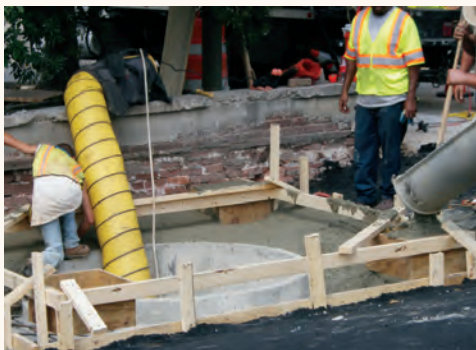
The MWA oversees a project to repair the storm drain on Pine Street in downtown Macon.
