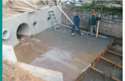
Storm water problem solved by MWA.
