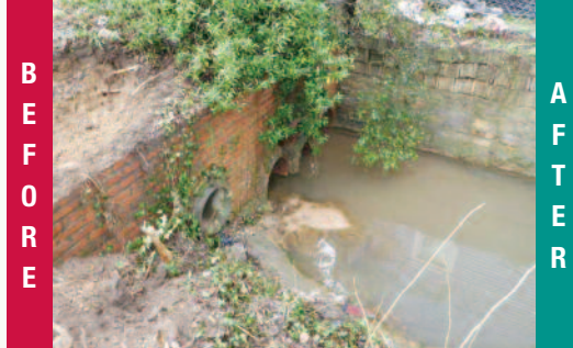
Storm water issue before project work by MWA.
